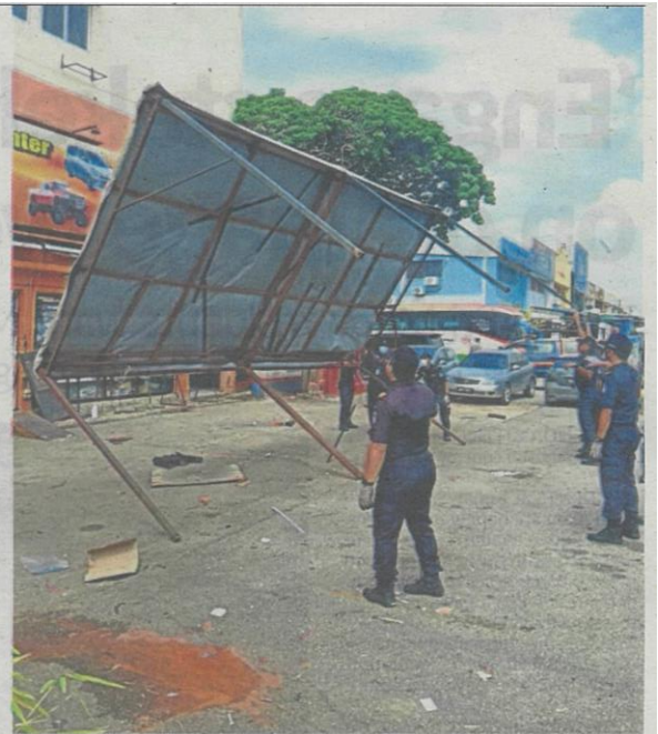
MPS enforcement team bringing down the canopy belonging to a car workshop, which had built the structure over several public parking bays.
